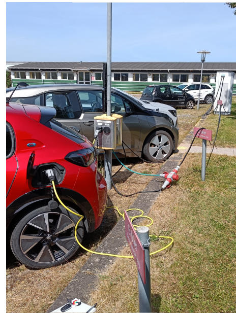
(b) Chargers on lightpole with one EV connected each.
