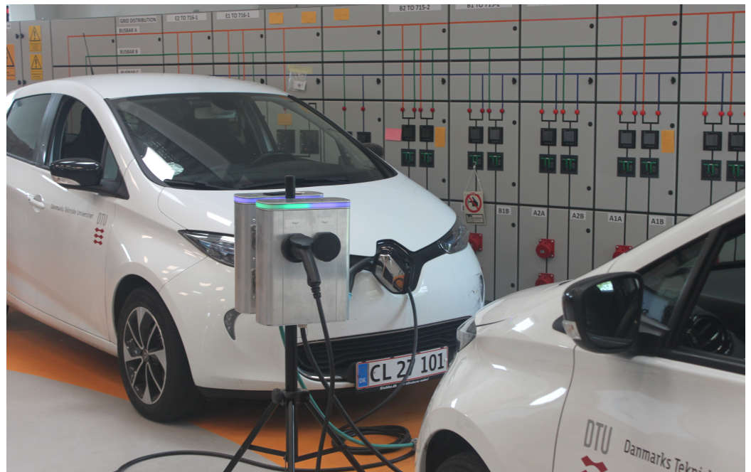
Figure 3. Experimental setup implemented: The figure shows the two Renault Zoes and the charger used in the test. The test is conducted in the DTU Energy System Integration Lab (SYSLAB).
