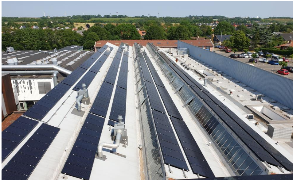
Figure 3 – The PV installation on Campus Bornholm
