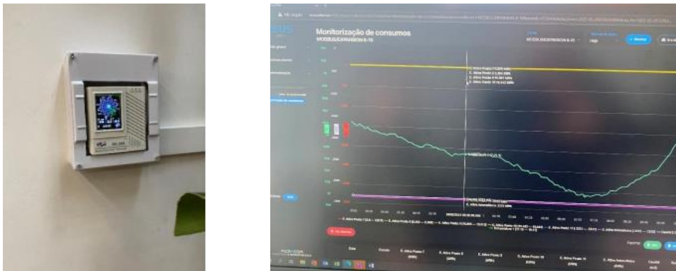
Figure 6 – EMS installed at LREC's office building: physical module (left) and visualisation dashboard (right)
