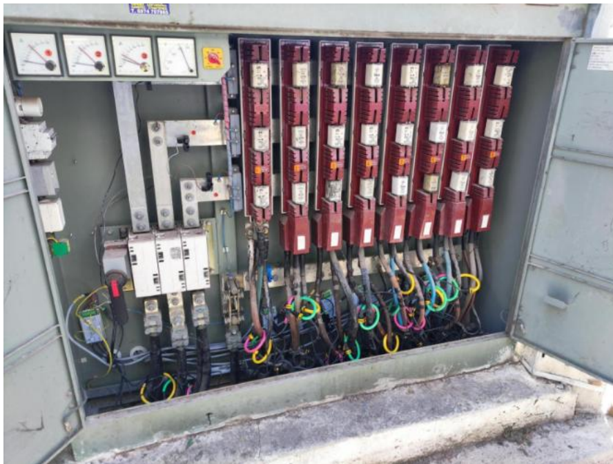
Figure 4: LV monitoring installation
