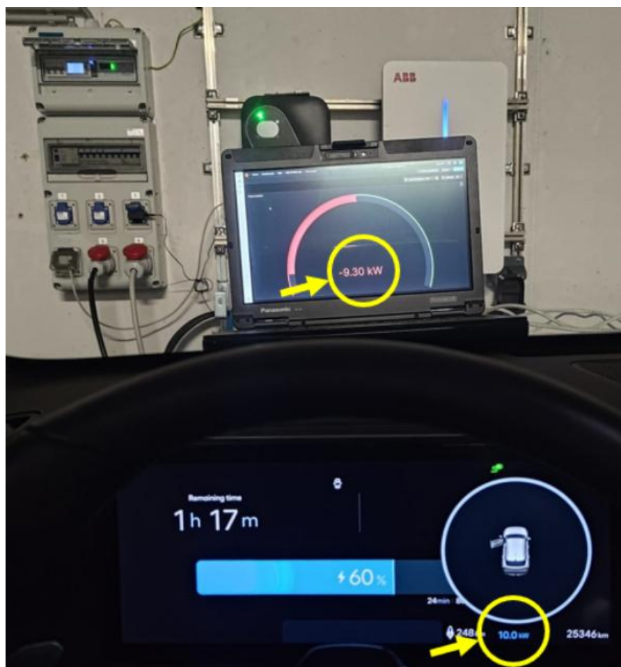
Figure 47: Discharging with ABB prototype CS
