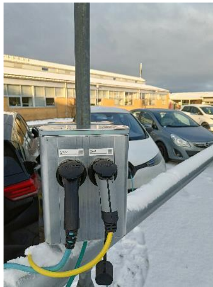
Figure 2: picture of one of the chargers installed in Risø campus
