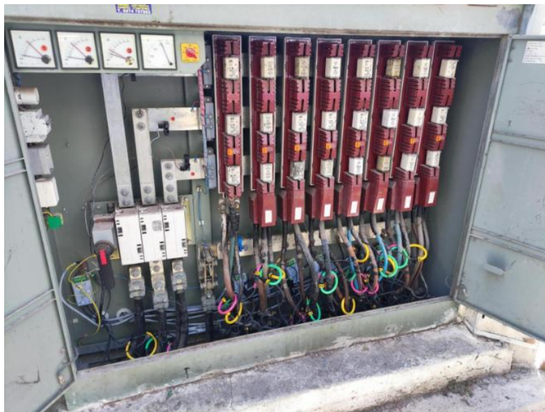
Figure 5: LV monitoring installation
